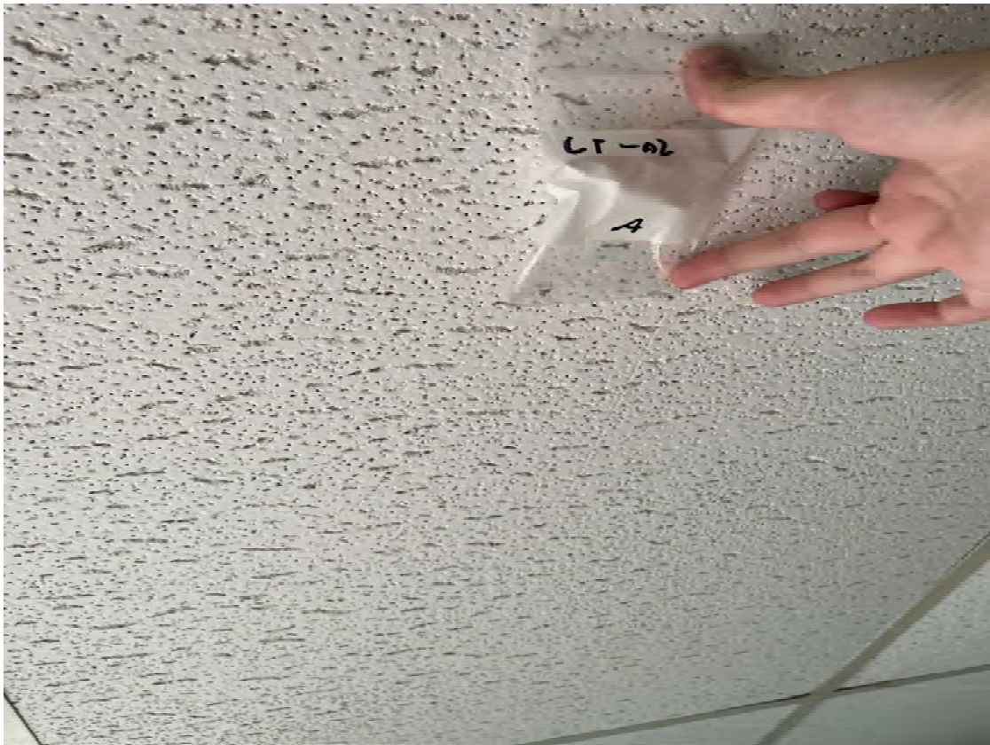
Upper Photo: CT-01-2' x 4' White Pinhole Ceiling Tile (Bldg. 1)
